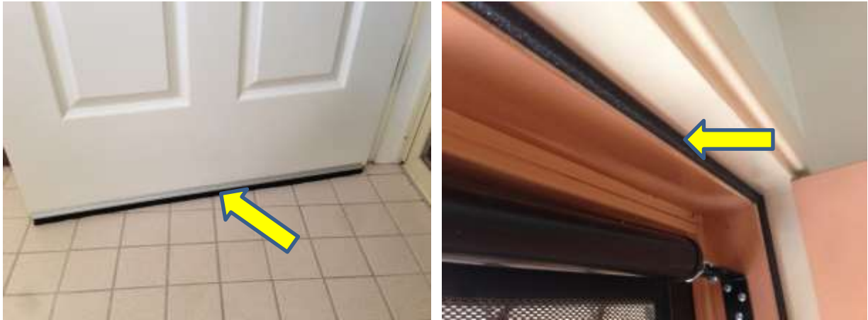
Figure 4.61 a) Typical door draught seal; and b) casement window draught seal retrofits.
