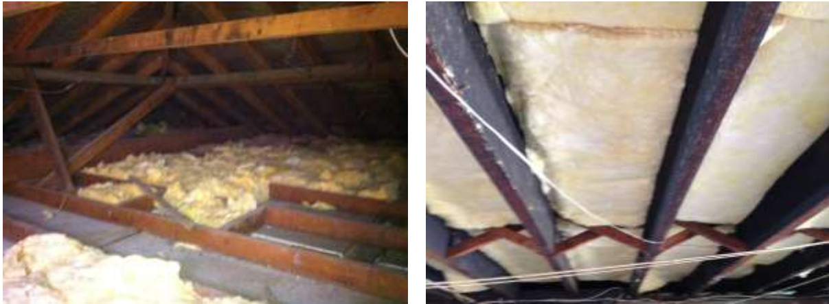
Figure 4.49 Typical examples of: a) ceiling space prior to insulation retrofit; b) completed underfloor insulation retrofit.
