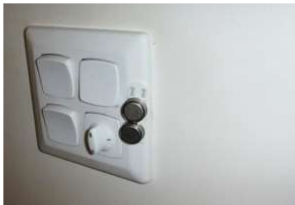
Figure 4.5 Typical installation of iButton temperature sensors to monitor living room temperatures.
