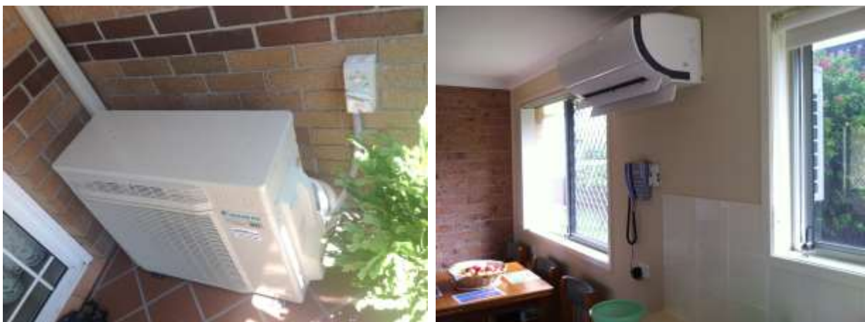
Figure 4.63 Reverse cycle air conditioning retrofits.
