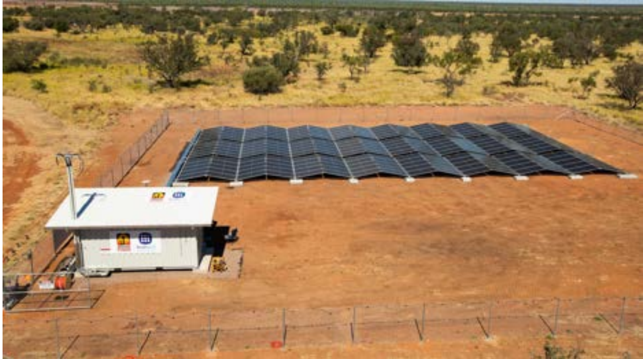
Image: Marlinja Community Solar Microgrid, commissioned July 2024.
